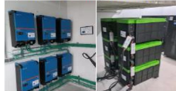
Batteries storage (80.64kWh)
